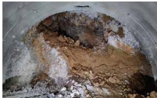
Fig. 3: Excavated tunnel face of the top heading in main tube at km 12+956 (left); the view from the First chamber towards main tube, big collapsed blocks can be seen on the floor (right; courtesy of: M. Prelovšek)
