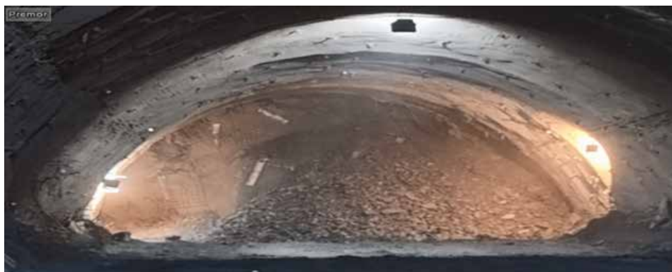
Fig. 13: Izkopno čelo kalote po dinamičnem zrušku dne 13.08.2023, ki ga je spremljalo intenzivno rušenje krovninskih plasti tektonsko močno poškodovanega in zdrobljenega meljevca. Excavation face of the top heading after the dynamic collapse on 13/08/2023, accompanied by the intense failure of the overlying layers of tectonically heavily damaged and crushed siltstone.
