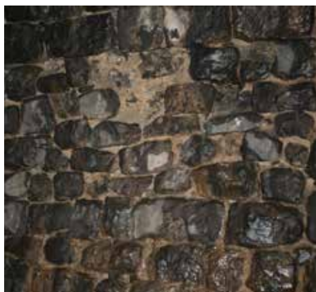
Slika 5: Stanje obloge, izpadanje kamnitih blokov (levo) in predhodna sanacija (desno) Condition of the lining, dislodging of stone blocks (left) and previous rehabilitation (right).
